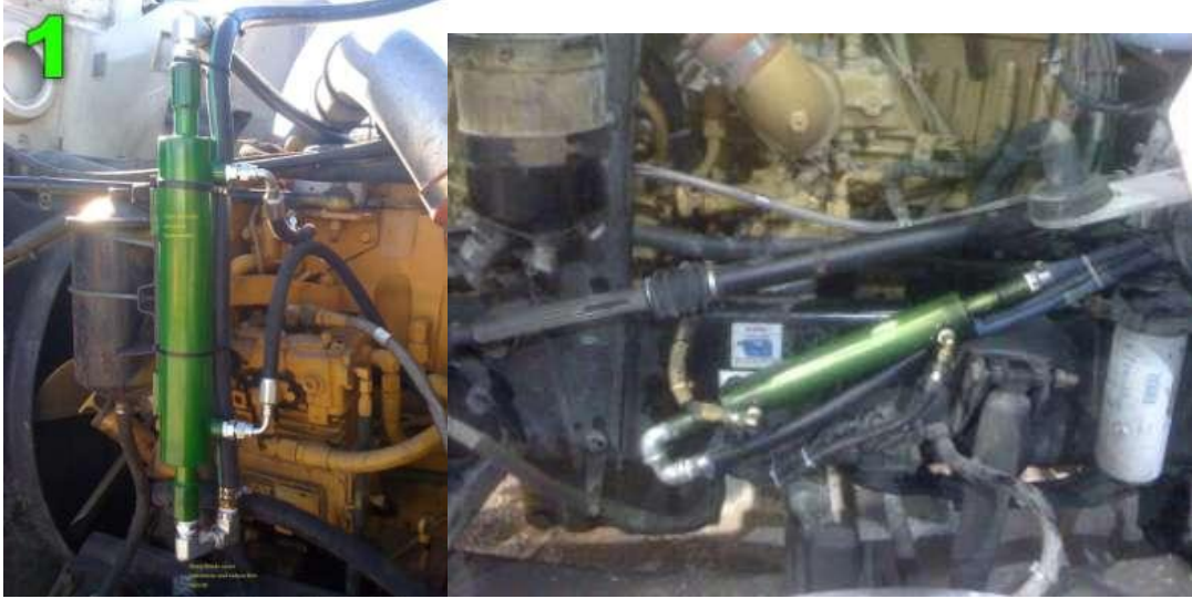
Pictures of IMPROPER mounting and coolant plumbing.
